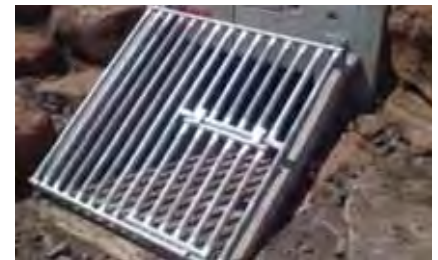
Example of a pipe grille installed on site
