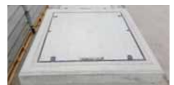
Concrete-encased and infilled access cover for an electrical pit
